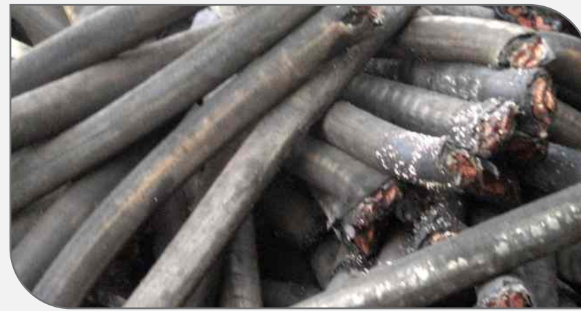
Relay ( Copper Lead) Cables
