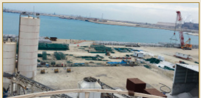
Design, Dredging & Construction of Berths 10 & 9 (& extension of Berth 1) - Ras Al-Khair Port, Saudi Arabia for SEAPORTS Authority (SEAPA), Kingdom of Saudi Arabia.
